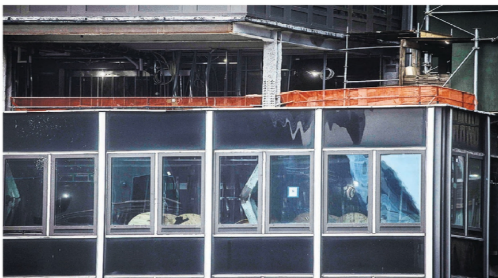
Pieces of a Midtown Manhattan office building began to crack and crumble as work was being done to convert the space to housing.
